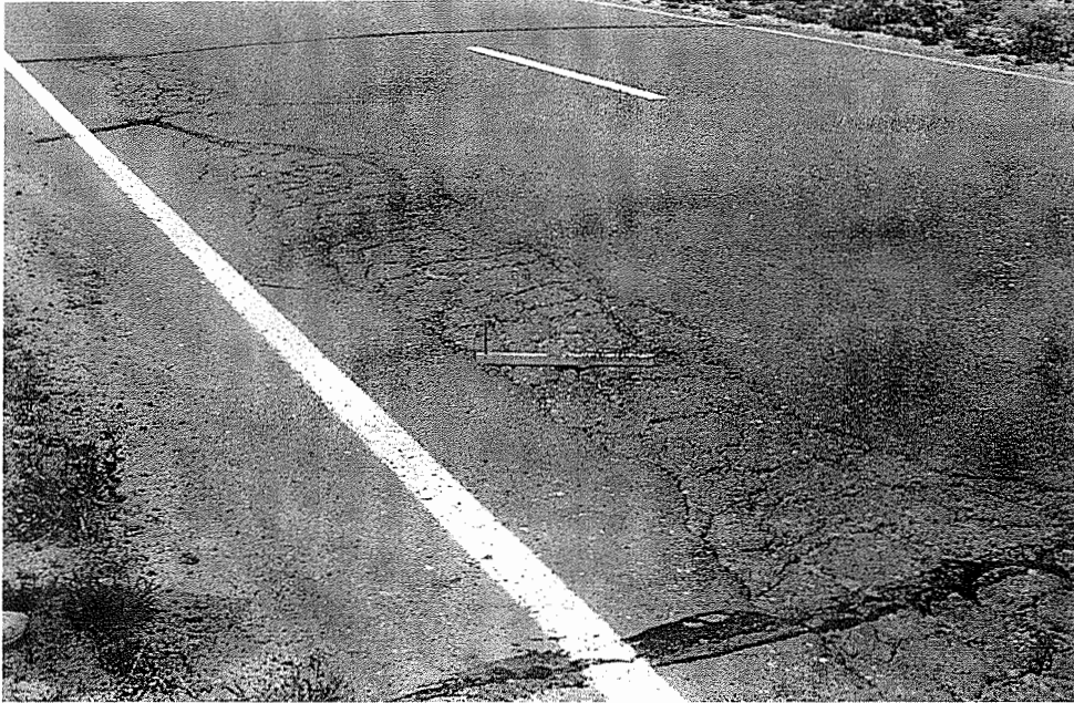
FIGURE 7 Fatigue cracking indicating weak pavement structure (Not candidate for preventive maintenance)
