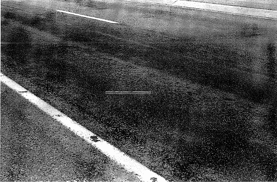
FIGURE 9 Bleeding (Candidate for preventive maintenance)
